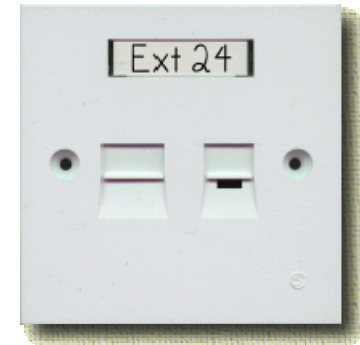
Data Wall Port
