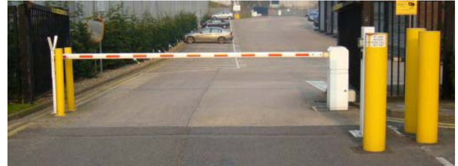
Automatic Traffic Barriers
